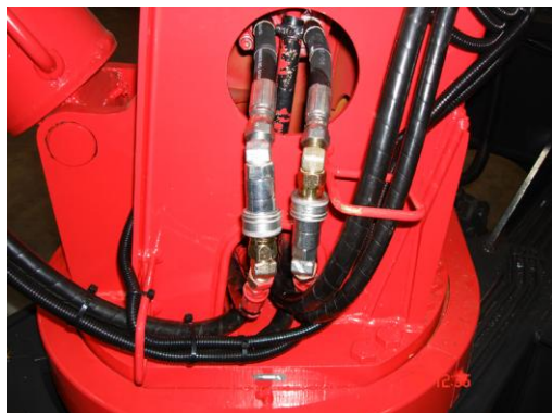
Illustration 4 showing pipes connected for normal crane winching operation
