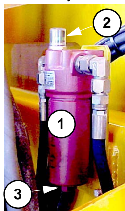
Photo 15 Hydraulic oil filter lateral movement circuit
